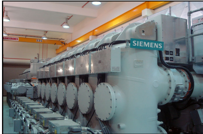
FIGURE 12.2: GAS INSULATED SUB-STATION
