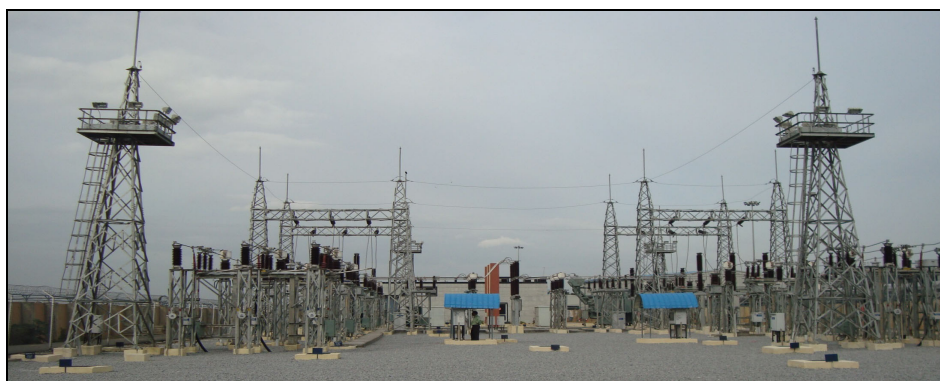
FIGURE 12.1: TYPICAL HIGH VOLTAGE RECEIVING SUB– STATION
