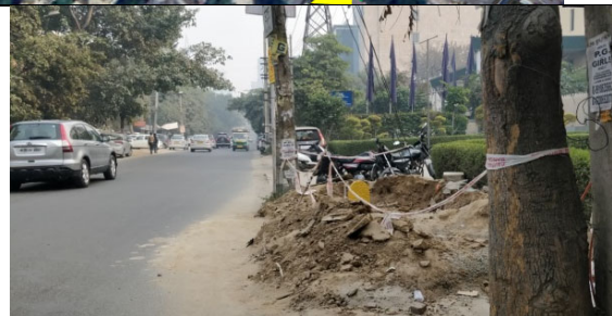
2. Lack of Continuous footpaths results in pedestrian spill on carriageway
